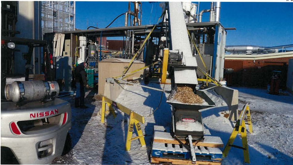
Figure 4. The conveyor used to carry the wood chips to the top of the gasifier.
