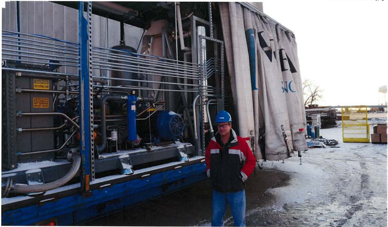
Figure 5. The gas compressor and gas-to-liquid reactor.
